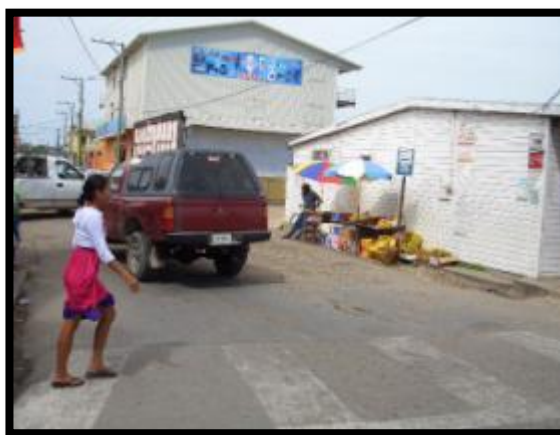
Pedestrian crossing showing fading of white areas
