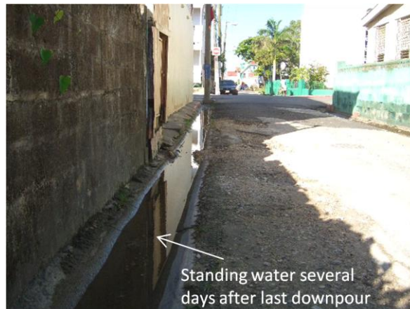
Belize City: Standing water in side drain (due to blockage and/or inadequate gravity)
