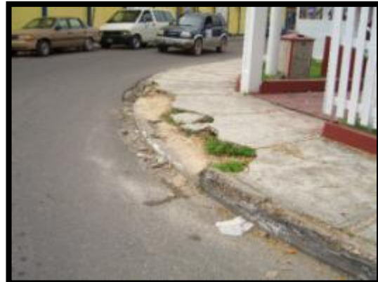
Broken Pavement at Downtown Area (most likely caused by heavy vehicle turning)
