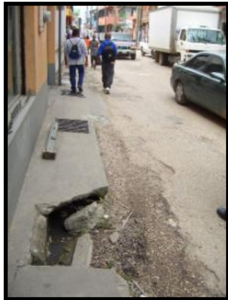
Poor Sidewalk Condition in Orange St (Central Area)
