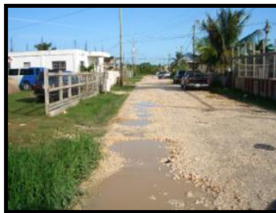
Belize City: Typical Suburban Street with Poor Gravel Surface and Drainage
